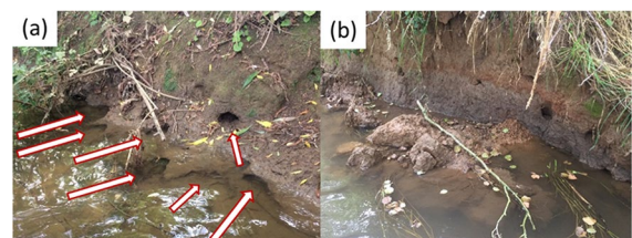
Fig. 1 Burrows constructed by signal crayfish in the UK. a Burrows in Gaddesby Brook, Leicestershire, UK, and b bank collapse facilitated by crayfish burrows on the River Bain, Lincolnshire, UK. Visible burrows in a are highlighted by the red and white arrows
